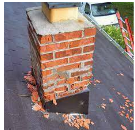
Example of damage from water
